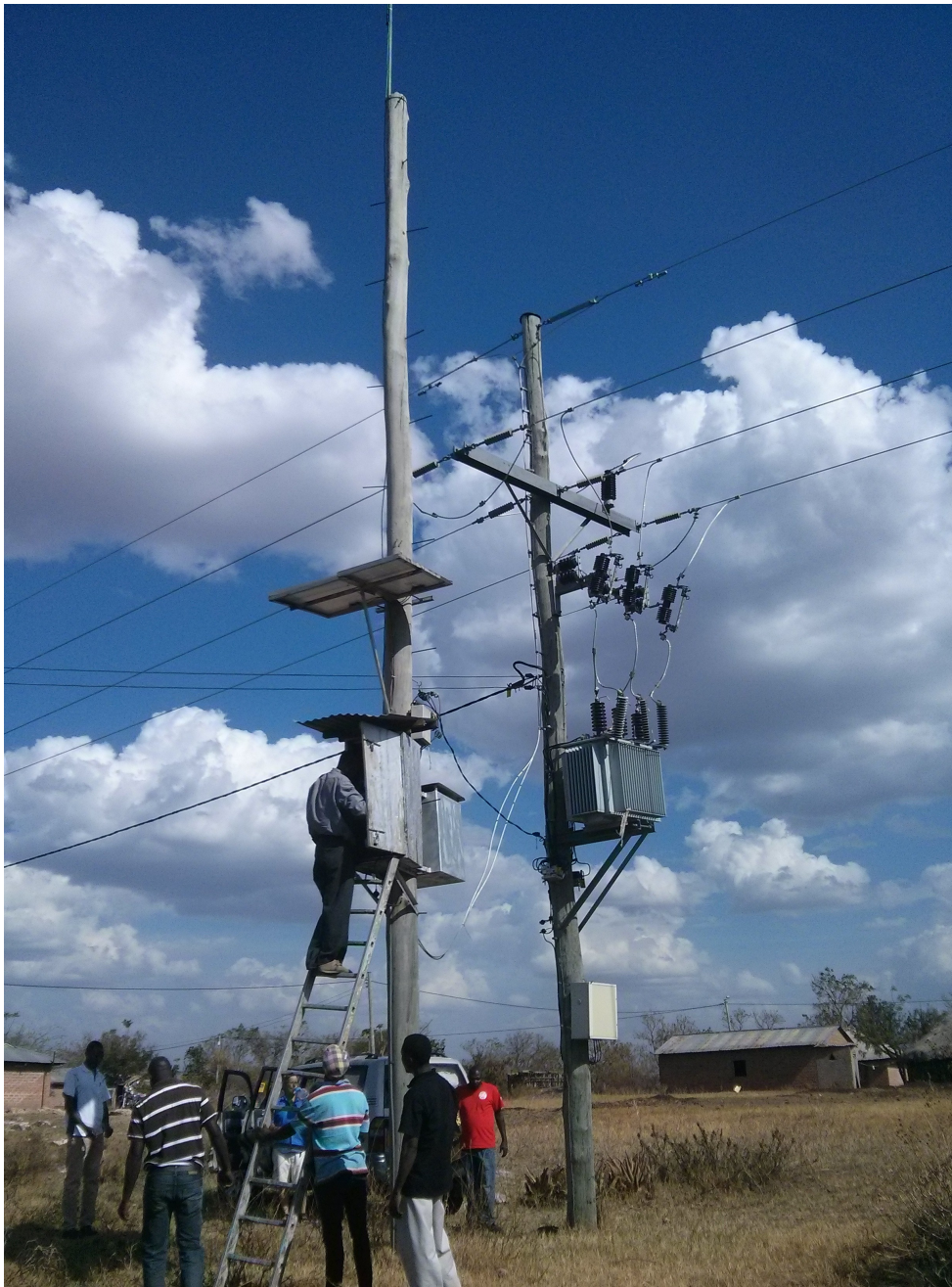
Serengeti Broadband Network node in the Nata Village, Serengeti District, Mara, Tanzania
