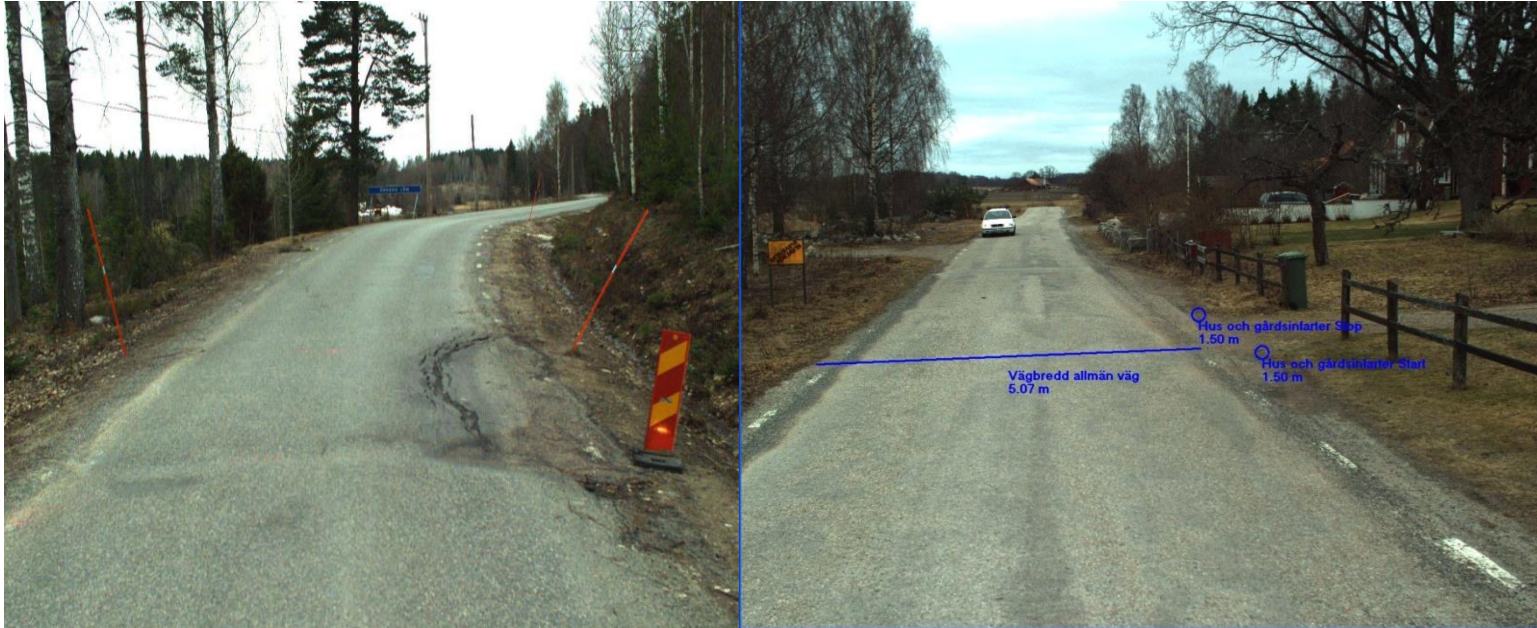
Inspection of damages
