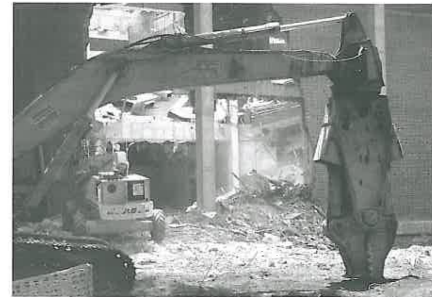
FIGURE 9.1 Partial demolition of the University of Florida Law School Library for a building expansion project. Truly green buildings of the future should be designed for deconstruction to maximize the reuse and recovery of building components and materials. (Photograph: Michele R. Moretti.)
