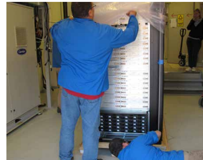
Above: The crates are removed before the racks are taken into the computer hall. See cover image for getting up the stairs!
