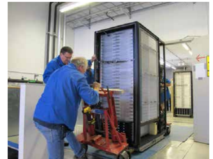
Above: Each rack is moved into the computer hall using metal sheets to protect the floor and distribute the weight.
