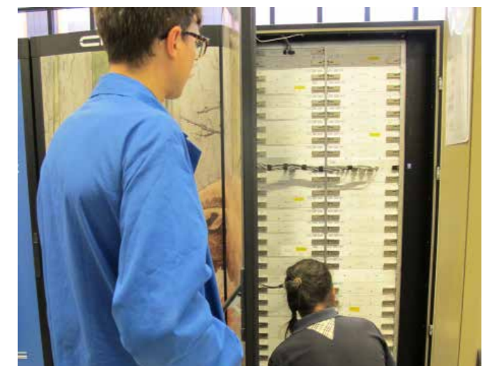
Above: Finally Cray staff and PDC staff work together to connect the new racks as part of the Beskow system.
