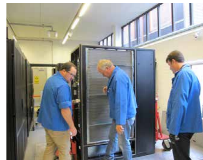
Above: It requires several people to move the racks to their final positions.
