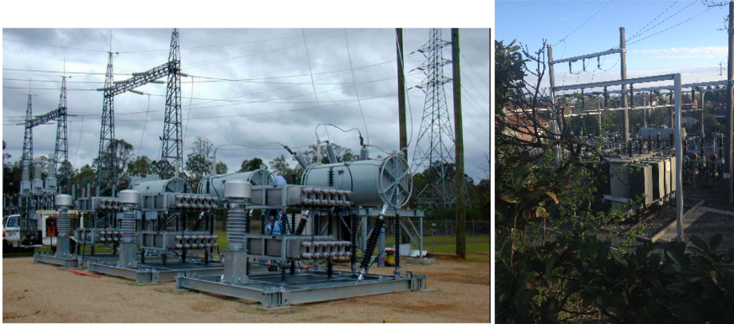
Figure 1: Capacitor bank and power transformer to step high voltage down to a safe level.
