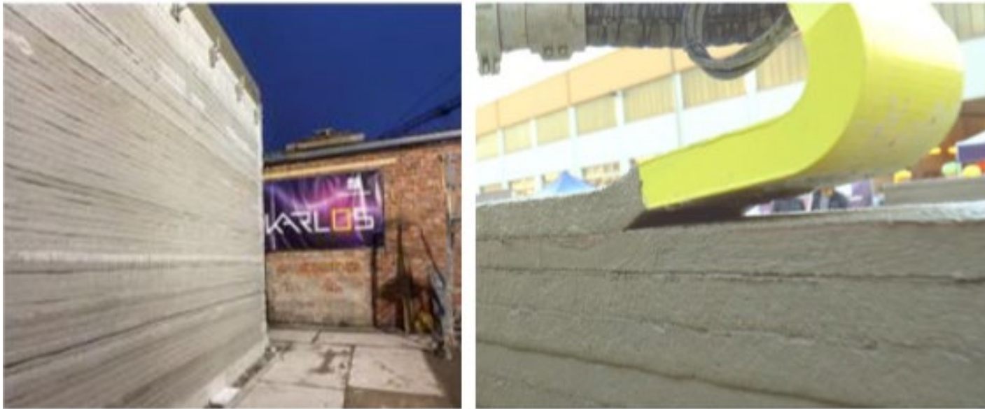
Fig. 2. Karlos printed structures a) 24-cm wide layers being printed, b) a printed wall.
