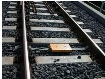
Figure 1. "Eurobalise" transceiver, installed between rails.
