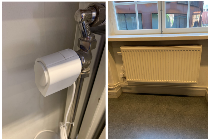
Fig 6 & 7: The thermostatic radiator valve (left) and the radiator in its context (right). 11
